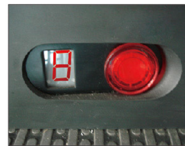
Fault Display for S and F Type
