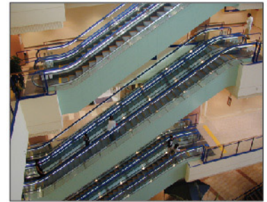
Light Under Handrail
